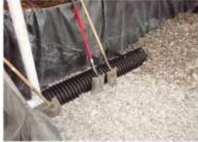
Influent distribution pipe (partially covered). Pipe from septic tank enters at bottom left.
