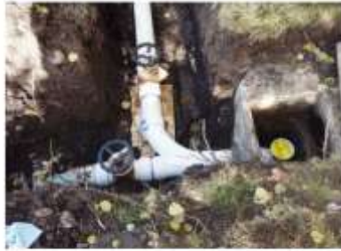
Pipe to RVF wetland (top) from septic tank (right). Preexisting pipe from septic tank to leachfield runs from right to left.
