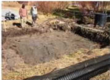
Excavation of RVF wetland cell. Groundwater level is at base of cell (center right). Pump vault is large vertical pipe at right.
