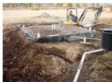
RVF wetland filled with gravel. Pipe at bottom is overflow from pump vault to leachfield.
