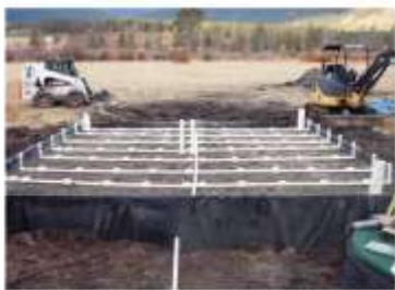
Recirculation distribution pipes installed at 6 inch depth. Pipe from pump is at bottom center.
