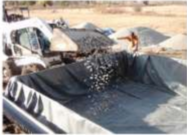
Filling lined RVF wetland cell with gravel. Gravel size is graded vertically from a coarse base to a fine root zone.
